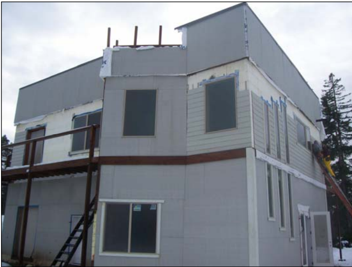
Platinum Development Northwest is constructing this single-family home in Shelton using energy efficient siding and heating.
